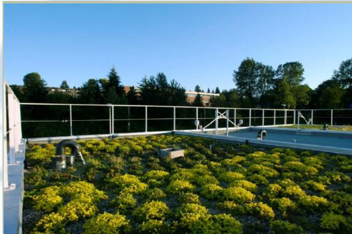
Green Roof Research Facility, Vancouver, BC, Canada
